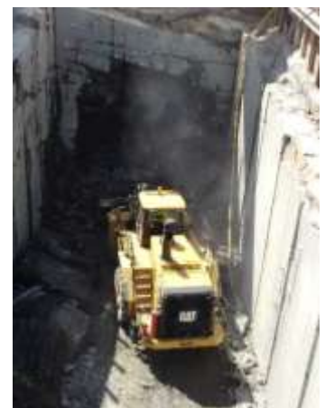
VSM are contracted by Implenia to unload the Varberg tunnel, which is a part of the West Coast Line rail link.
